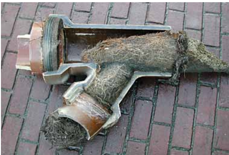
Figure 6. Although tree roots commonly grow into sewer pipes through breaks and loose joints, they are rarely the cause of damage to pipes.
